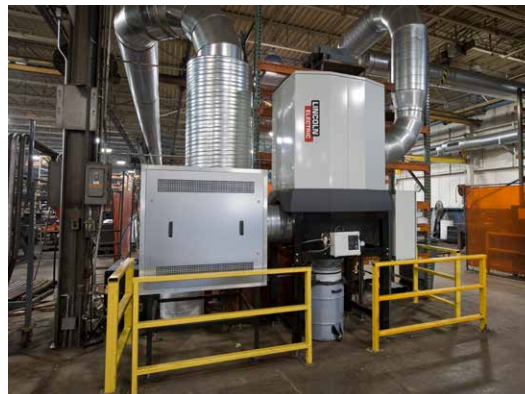
Push/Pull System installed at Elgin Sweeper Company
